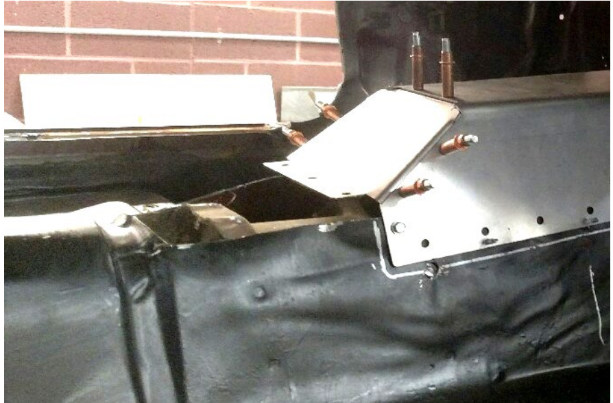
Figure 7: Gap between the floor and tunnel cover
